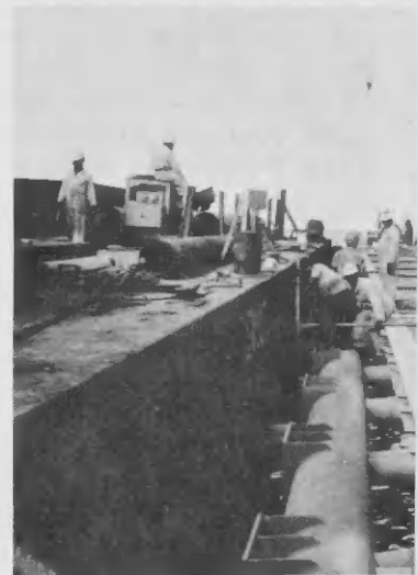
Above, progress is underway on the West Pier. Job required twenty precast concrete slabs to be removed through the use of a crane and barge. Ariba, trabao ta den progreso ariba e barge aki ta requeri bini
